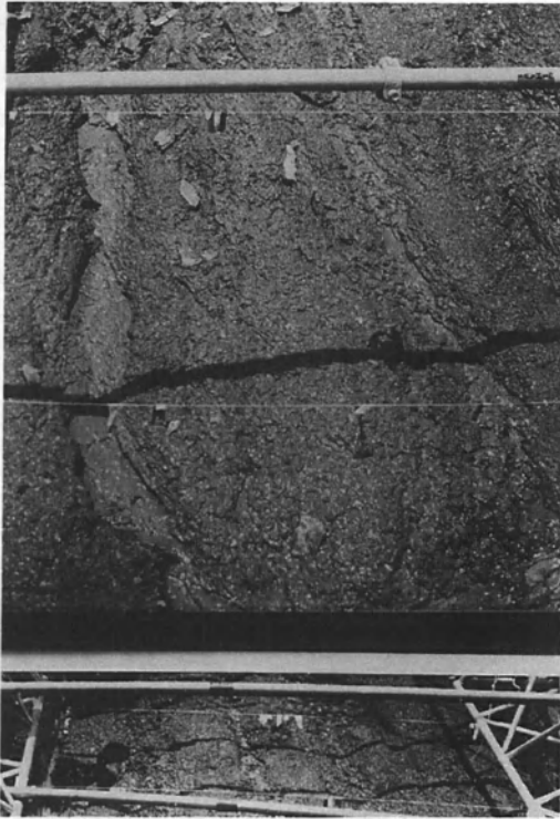
▲ Large rills on slope A
